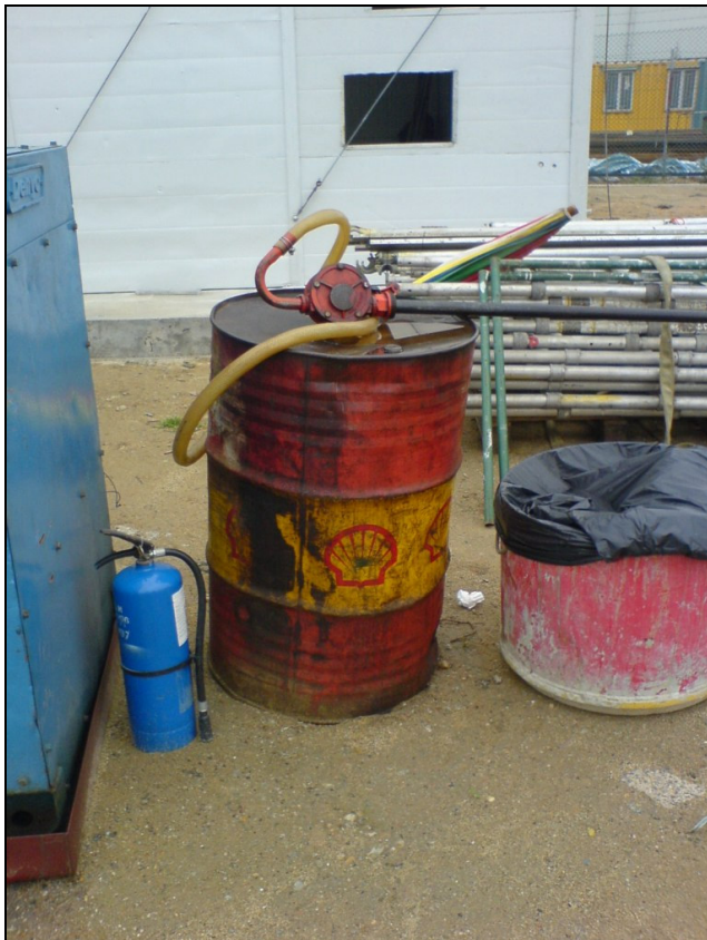
Photograph 8-2 No drip tray was provided to the oil drum in EP07-03
